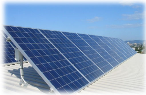
Traditional Solar Panels
